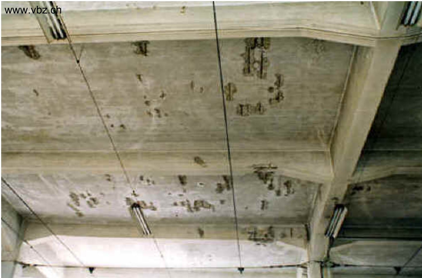
damage of concrete
